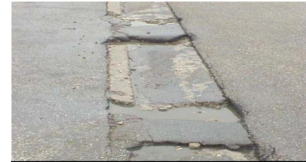
EXAMPLE: Large Holes in Surface
